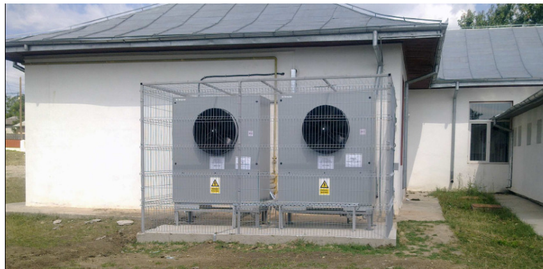
Fig. 2 – Front view of the air-to water heat pumps.
